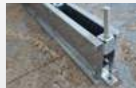
The racking is fixed to the floor using M10 x 90mm anchor bolts.
